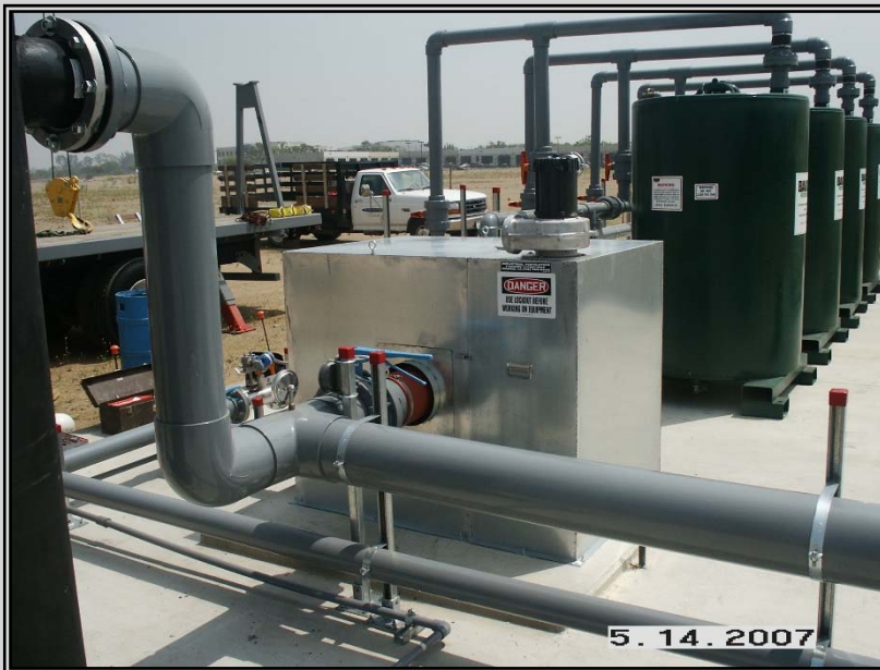
FanAir Co. 6 Ft x 6 Ft x 5 FT Fiberglass Acoustic Sound Enclosure designed and built for a Fiberglass Odor Control Blower for a Biofilter Located in Orange, County, Ca.
